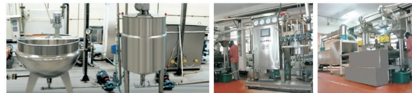
化糖锅和储糖锅 Sugar dissolving cooker and storage tank
